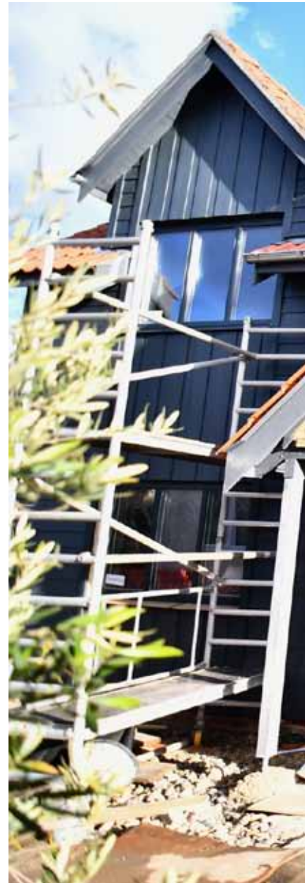
ABOVE: Trevor and Dee Taylor’s Svenskhome is under construction at Ashfield Green
